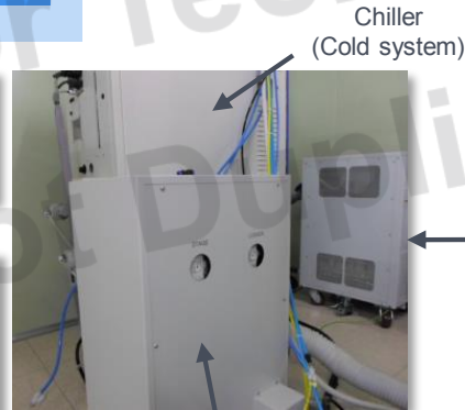
Air dryer system
